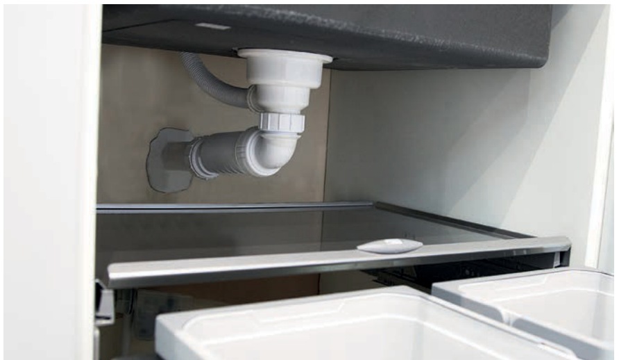
Figure 3: Space saving capabilities under a kitchen sink
